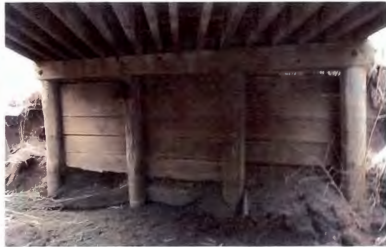
Abutment 2(N) timber backwall condition
