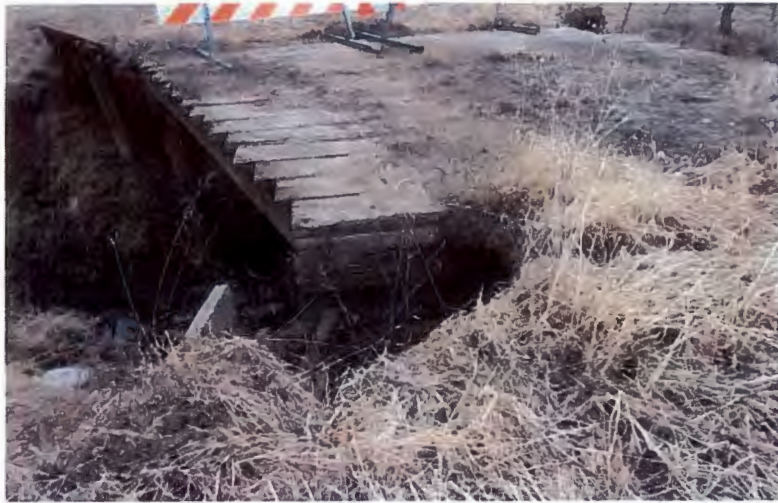
NE corner erosion
