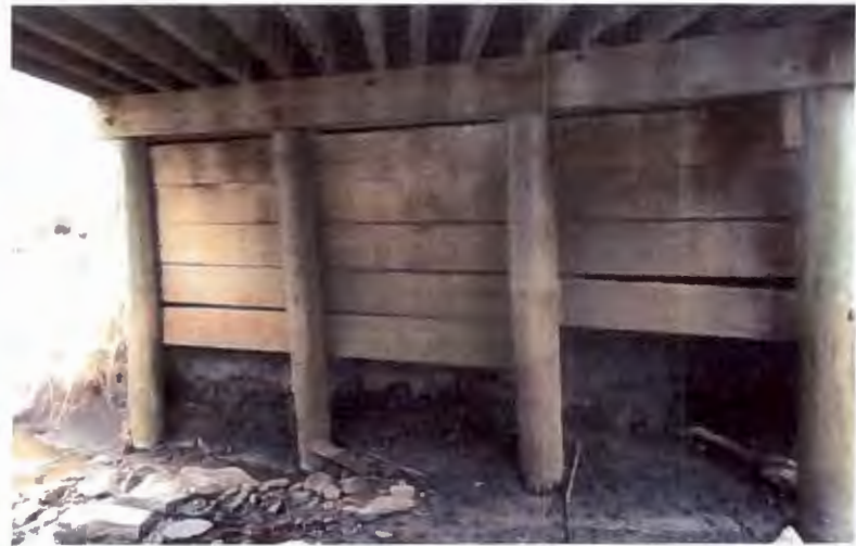
Erosion at Abutment 1(S)
